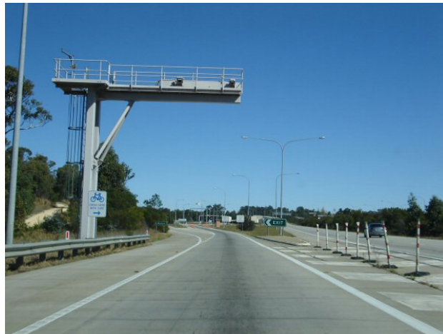
Photo 8.1 Automated enforcement gantry approaching Marulan weigh station, NSW.
